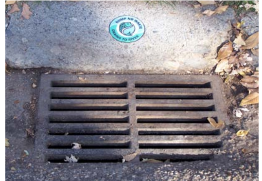
A marked storm drain.
